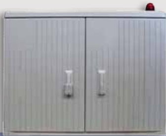
External cabinet with flashing light
